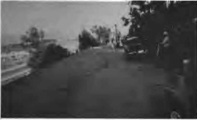
Figure 2. Crack along berm road, northside of the OII landfill.
