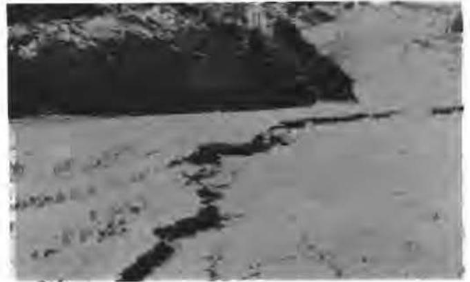
Figure 5. Crack along top deck at the western end of the Sunshine Canyon Landfill (Photo courtesy of Calif. EPA, Integrated Waste Management Board).
