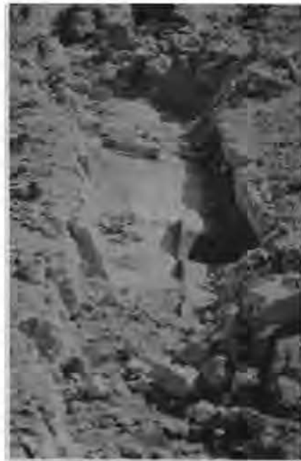
Figure 4. Tear in the HDPE geomembrane liner system, Canyon C, Chiquita Canyon Landfill (Photo courtesy of Calif. EPA, Integrated Waste Management Board).
