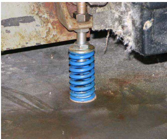
Fig. 18. The new system of isolation for the raper type weaving looms.
