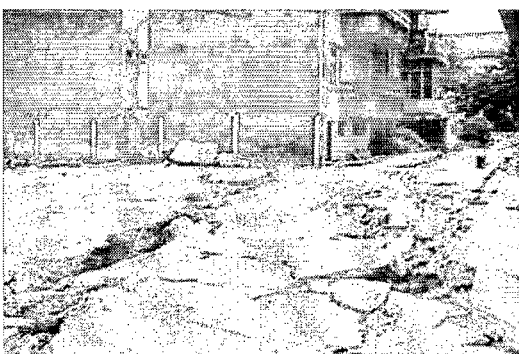
Fig. 9. Damage caused by large ground fissure
