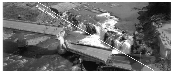
Fig. 1. Collapse of two spans of the Bei-Fung bridge due to tectonic dislocation in the 1999 Chi-Chi (Taiwan) earthquake.
