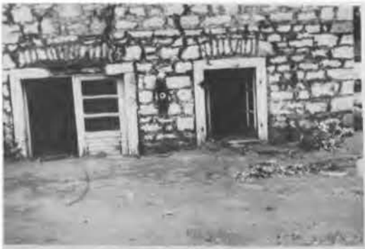
Fig. 4 Damage due to liquefaction: sinking of house and soil, house floor and its surrounding covered with outburst sand, cracks in the walls
