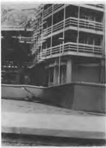
Fig. 3 Soil liquefaction consequences observed on the hotel and swimming pool structures
