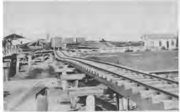
Fig. 21 Warehouse at Moss Landing Destroyed by Lateral Spreading in the 1906 San Francisco Earthquake [Lawson et al., 1908]
