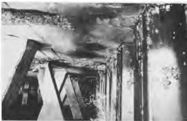
Fig. 14 Tensile Failures at Top of Battered Piles at the 7th Street Terminal [Photo courtesy of the U.S. Army Corps of Engineers, South Pacific Division]
