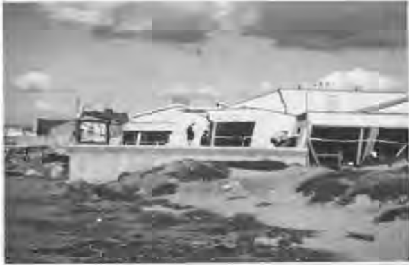
Fig. 20 Damage to the Moss Landing Marine Research Facility as a Result of Settlement and Lateral Spreading
