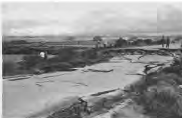
Fig. 18 Flow Failure of the Moss Landing Approach Road Embankment
