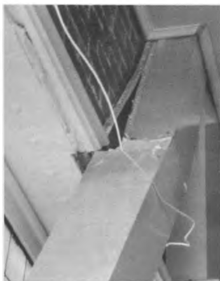
Fig. 16 Buckled Brace in URM Building
