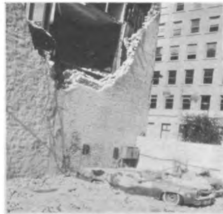
Fig. 7 Out-of-Plane Failure of Masonry Wall
