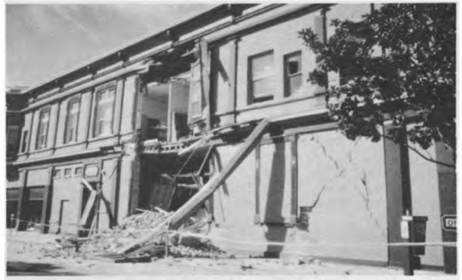
Fig. 9 In-Plane Failure of Masonry Wall
