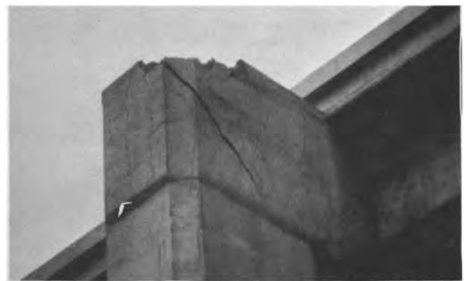
Fig. 25 Damaged Knee Joint in New Freeway
