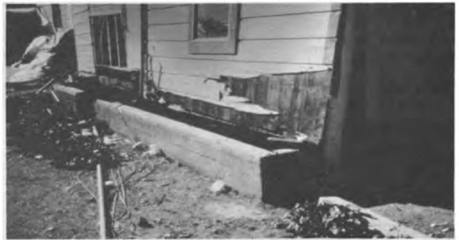
Fig. 2 Damage to House Not Bolted to Foundation
