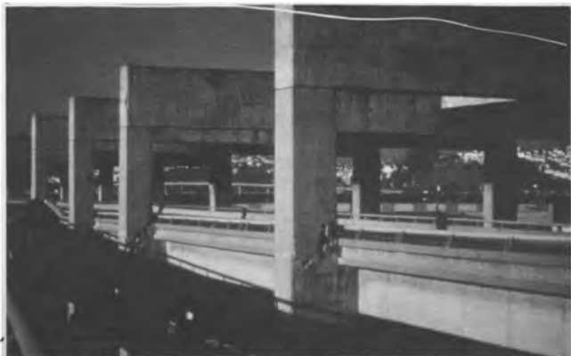
Fig. 24 Damage to Southern Freeway
