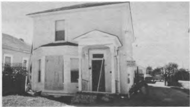
Fig. 4 Collapse of Home on "Pony" Walls
