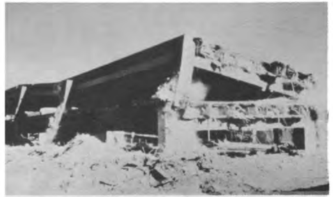
Fig. 23 Failure Mode Observed during Demolition
