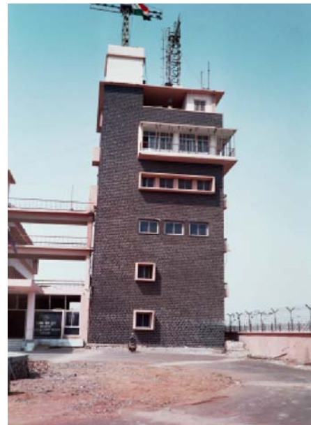
Fig. 1. Rotation of the HMT building at Kandla Port following the Bhuj earthquake
