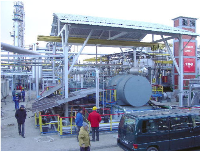
Fig. 1. General view of the compressor.
