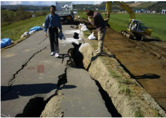
Fig. 33. Longitudinal cracks along river dike (Ushishubetsu River after 2003 Tokachi-oki earthquake ).
