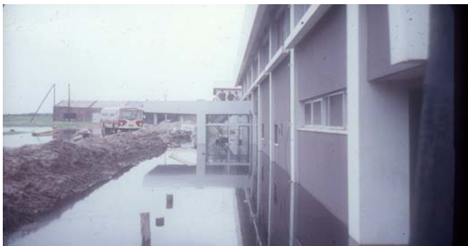
Fig. 28. Subsided shape of Niigata Airport Terminal Building (Department of Civil Engineering, University of Tokyo).
