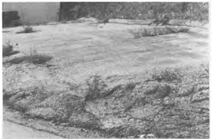
Figure 3b. Creep at Toe of a Sensitive Slope.
