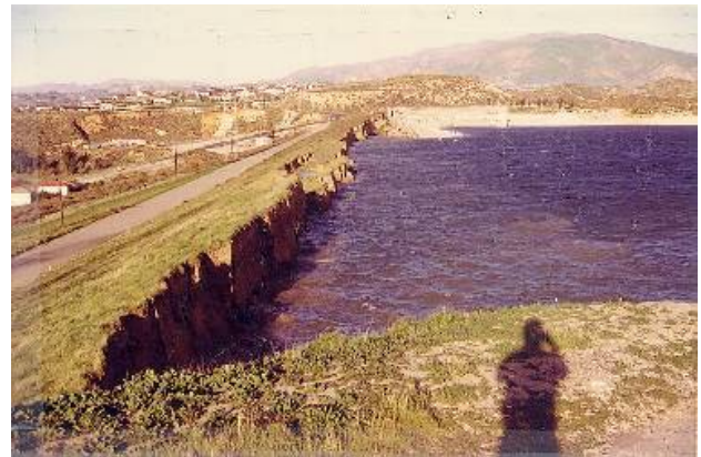
Fig.2 –San Fernando dam –upstream slope slide
