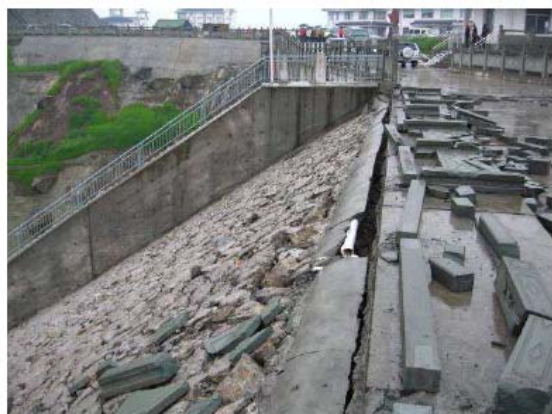
Fig. 14 Zipingpu dam crest damages (after Chen, 2008)
