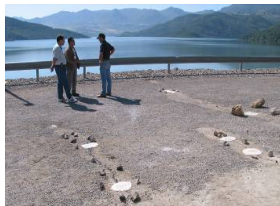
Fig. 6. Keddara dam-cracks observed at the crest
