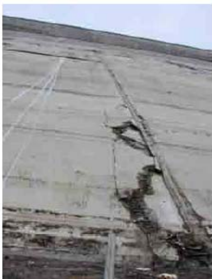
Fig. 15. Zipingpu dam joint damages (after Chen, 2008)
