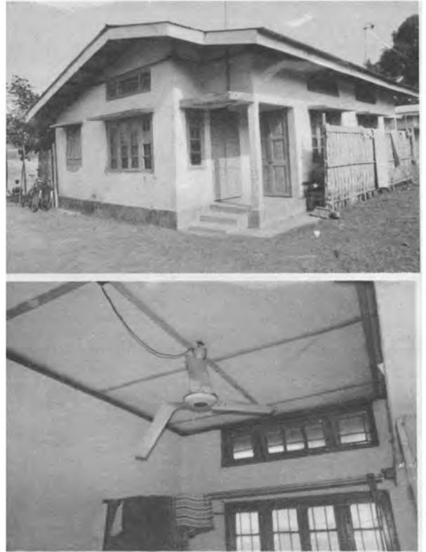
Fig. 2. Bending of blades of a ceiling fan in a building with reinforced concrete columns and beams, near the one in Fig. 1.
