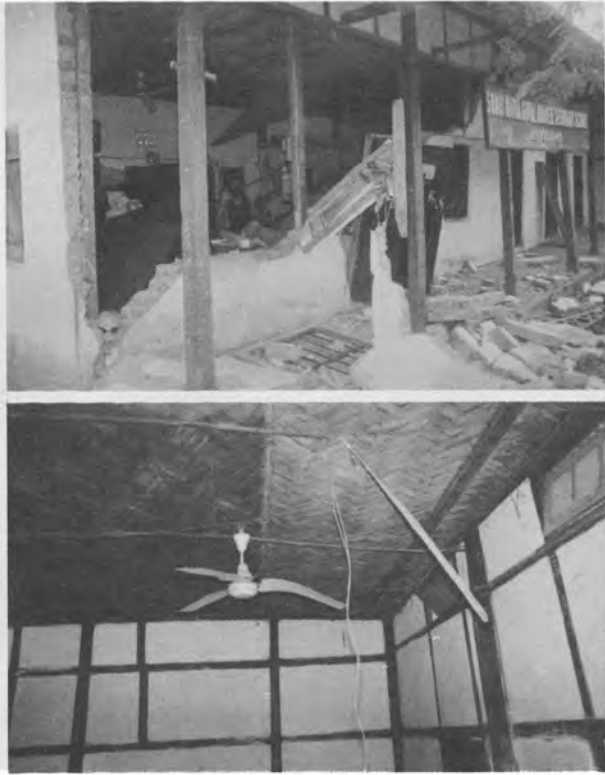
Fig. 1 Bending of blades of a ceiling fan in a timber frame building at Sonaimukh during Cachar earthquake.
