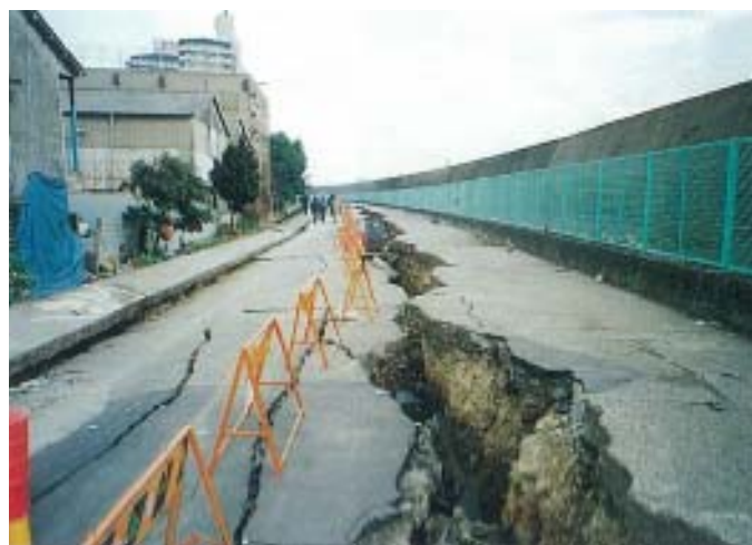
Fig. 36 Seismic damage to high tide protection wall in highly industrialized area during 1995 Kobe earthquake
