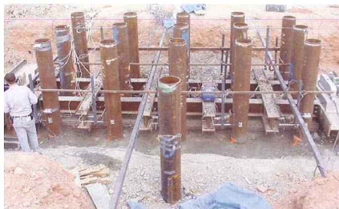
Fig. 24 Full-scale lateral load test layout; a reference single pile in front of 3 x 5 group pile(Snyder, 2004)
