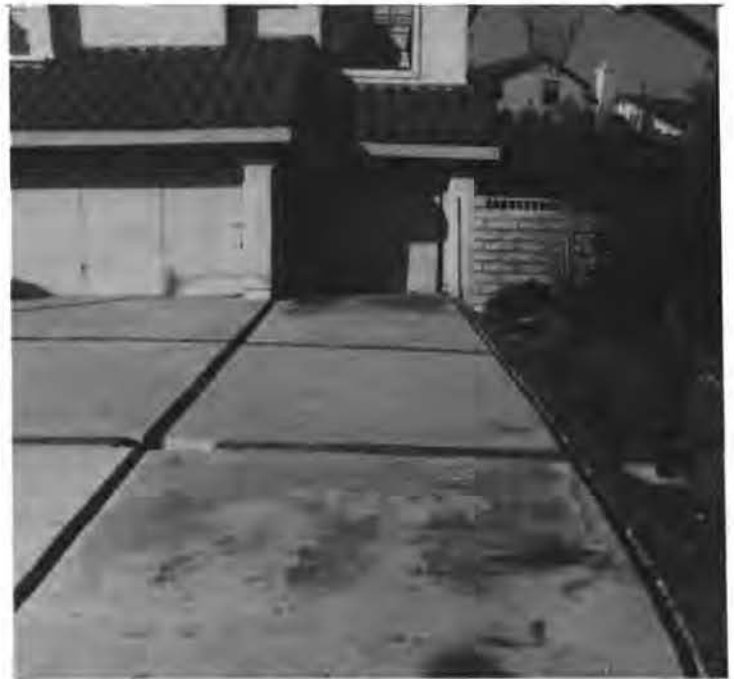
Figure 5: Typical crack at the cut/fill contact. The top of slope is visible on the right side of the photograph.
