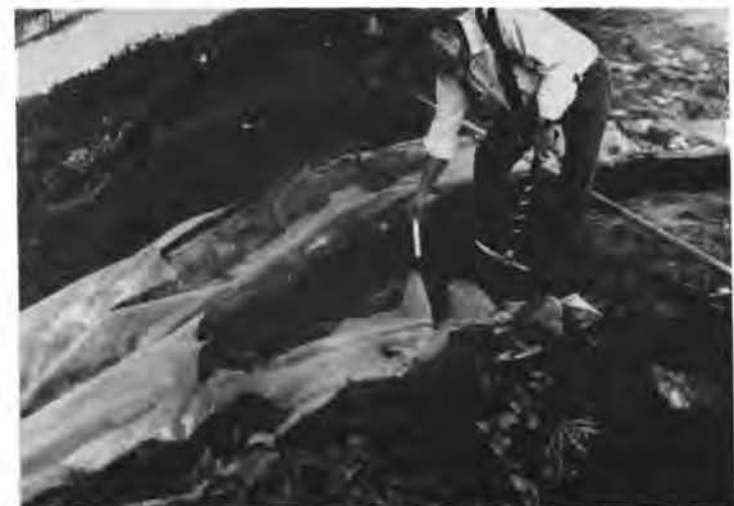
Figure 6: Typical down drain uplift, at one-third of the slope height up from the base of the fill (see also Figure 4).
