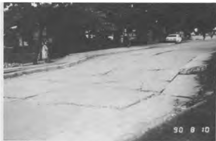
Photo 1 Surface faulting near Rizal
