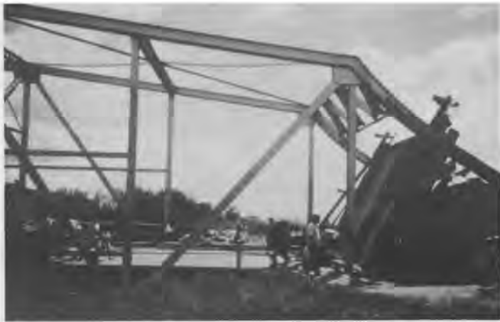
Photo 20 Carmen Bridge destroyed by lateral spreading due to soil liquefaction
