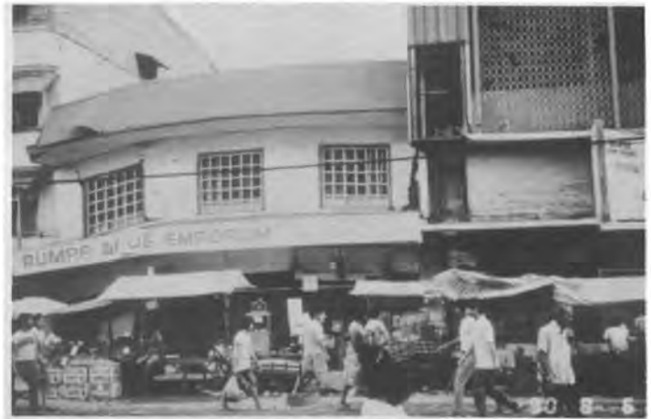
Photo 15 Damage to light-weight structure sandwiched in between heavier buildings
