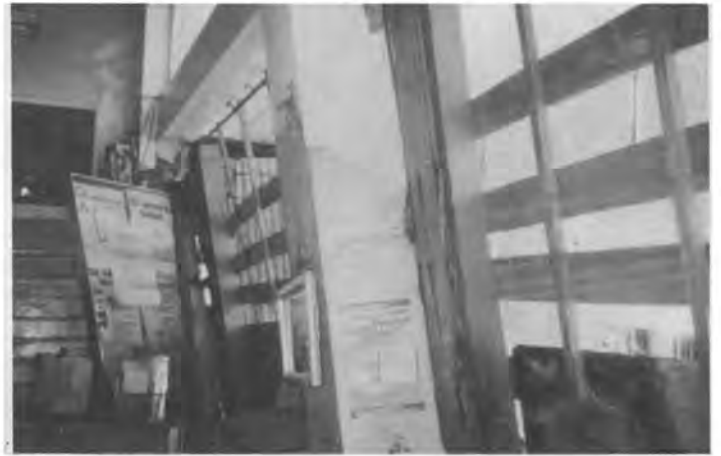
Photo 9 Inclined columns due to lateral movement of footings
