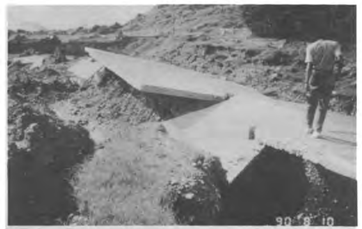
Photo 19 Damage to road near Rizal
