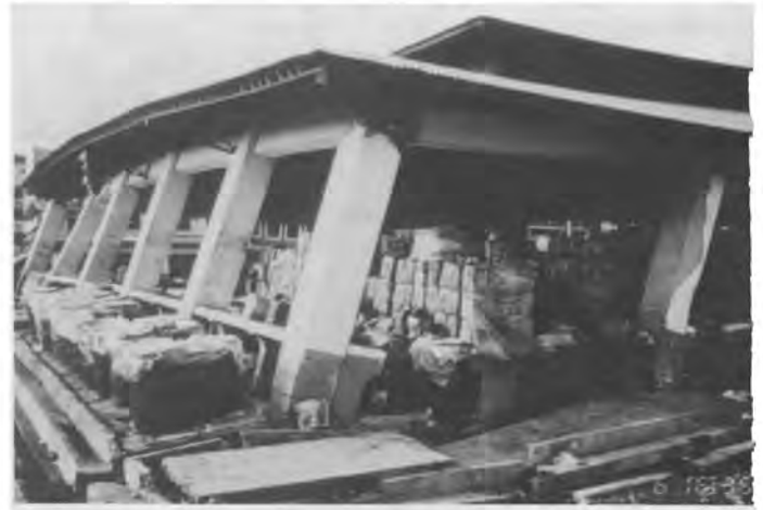
Photo 13 Warehouse in sliding area
