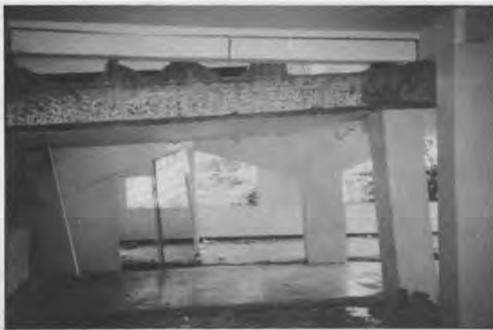
Photo 10 Significant differential settlement in two-storyed school
