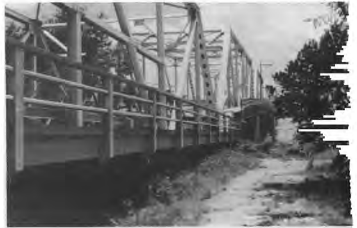
Photo 21 Damage to Carvo Bridge and lateral spreading of its foundation soil
