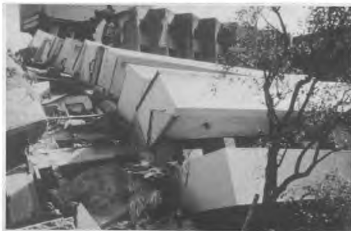
Photo 3 Pancake crush of a building in Baguio
