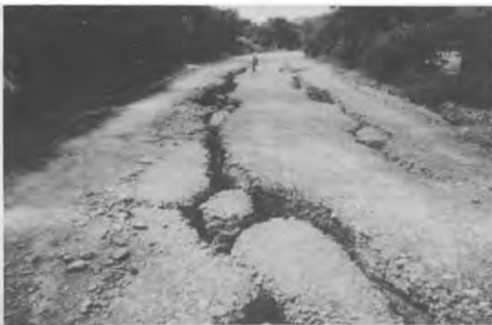
Photo 18 Large fissures near Rizal
