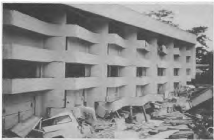
Photo 2 Soft first story failure of a building in Baguio
