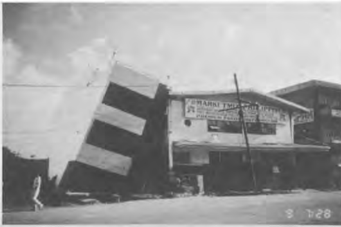
Photo 14 Damage to structure caused by overlying building
