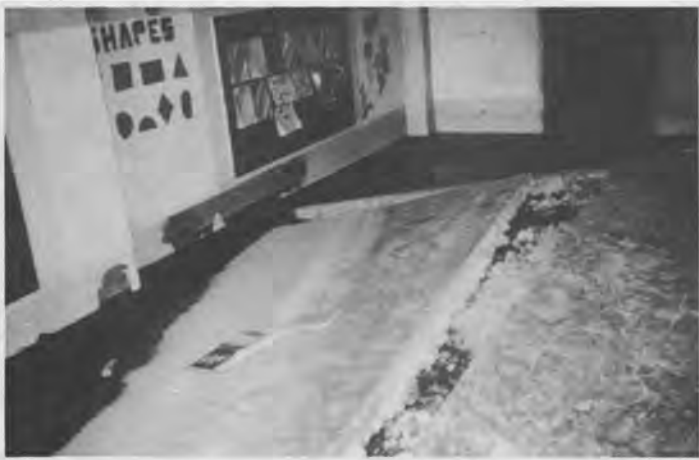
Photo 8 Heaved slab due to bearing failure of footings
