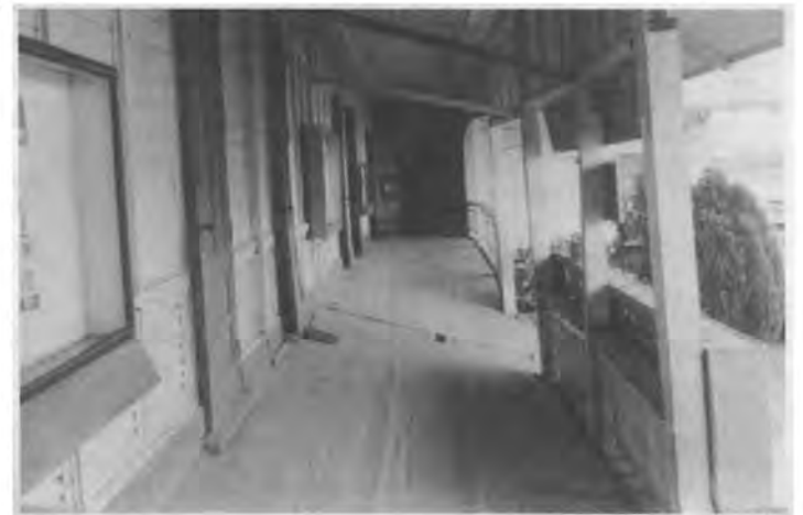
Photo 11 Differential settlement due to partial bearing failure
