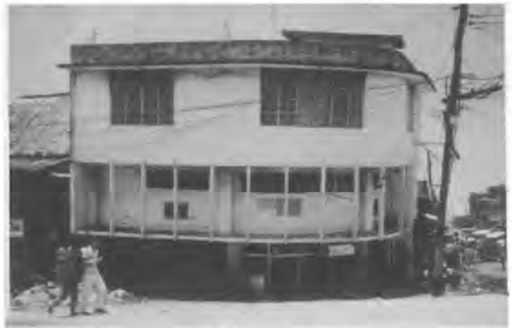
Photo 5 Bearing failure of three-storied building in Perez Blvd.
