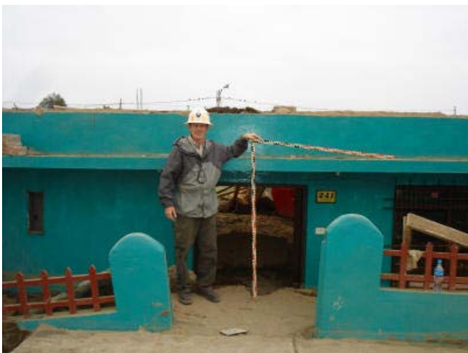
Fig. 6. Approximately 0.9 m of liquefaction-induced settlement at a one-story house in Tambo de Mora.
