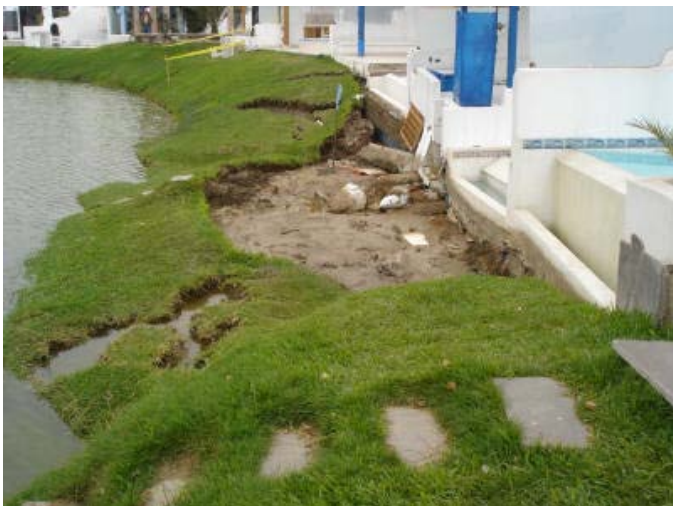
Fig. 4. Lateral spread with a displacement of 3.9 m. The house located in front of this lateral spread suffered considerable damage due to differential settlements.
