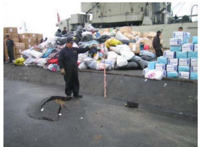
Fig. 7. Vertical displacements as large as 0.8 m were observed between the pile-supported wharf and the reclaimed
