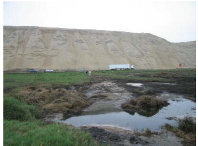
Fig. 5. A view of the Pan American highway at the location of the 400 m long Jahuay slope failure. Marine terrace deposits are in the foreground and the Cañete Formation in the background.
