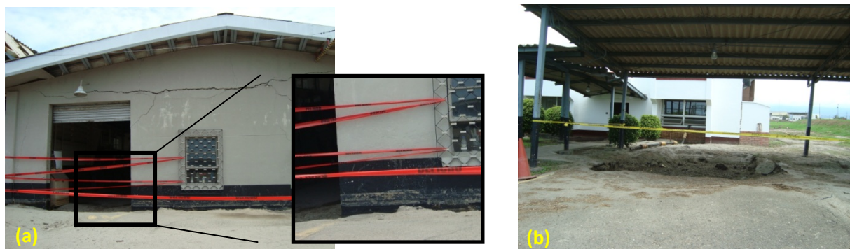
Figure 5 – (a) Buildings and small structures sank up to 3 ft and were flooded with liquefied sand [06/20/2009, 1:08 PM, N15.849851, W87.95793], and (b) vehicles sank into sand boils, see carport automobile was already extracted [06/20/2009, 1:25 PM, N15.848216, W87.958604].
