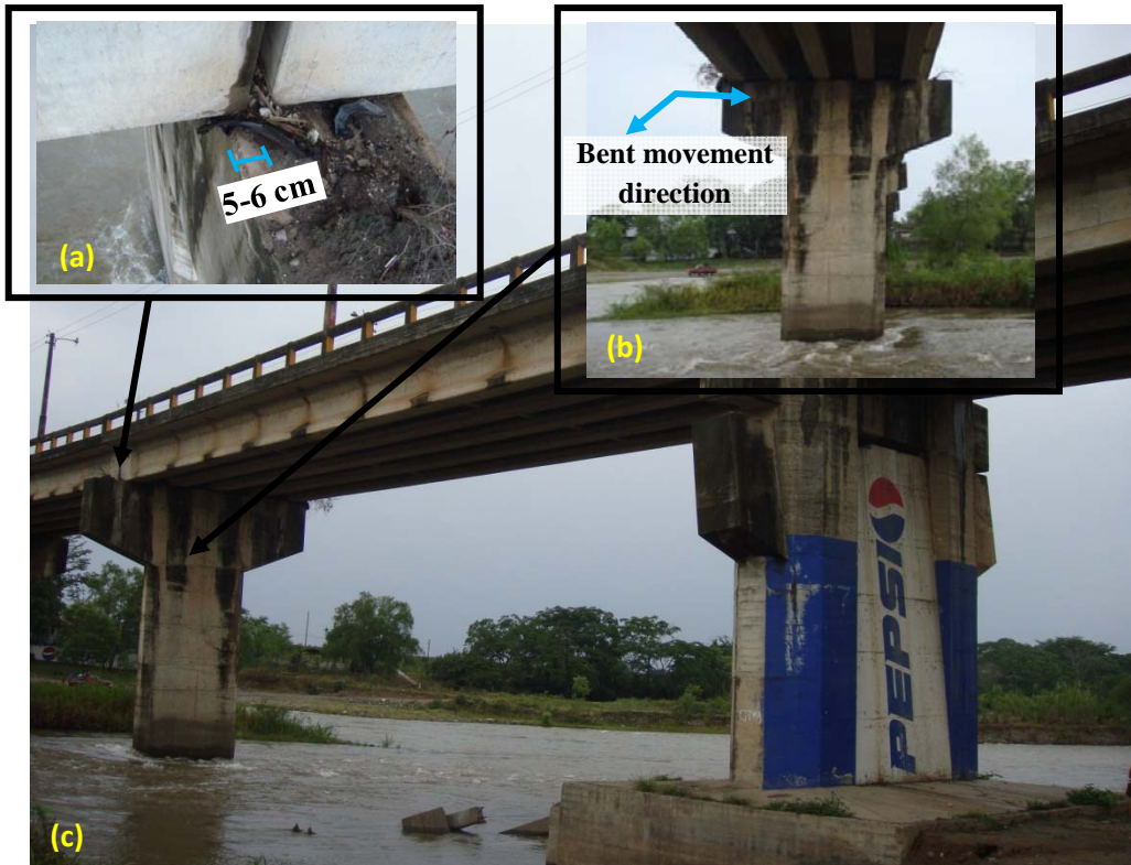
Figure 14 – Santa Rita Bridge over the Humuya River after the earthquake and before collapse (a) [06/21/2009, 6:08PM, N15.191548, W87.82559], (b) [06/21/2009, 5:43PM, N15.191017, W87.8922393], (c) [06/21/2009, 5:40PM, N15.190907, W87.892658]
