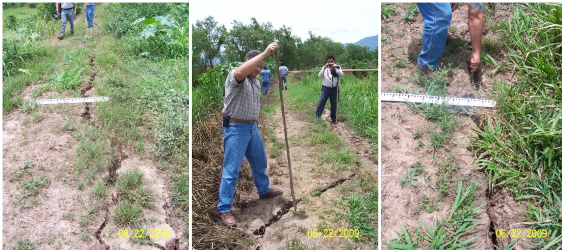
Figure 10 – Cracks at the crest of levees exceeding 1.5m deep [06/22/2009, 11:57AM, N15.344505, W87.868515].
