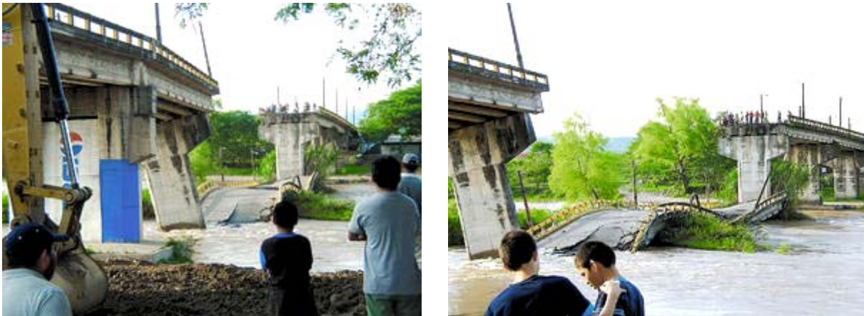
Figure 15 – Collapse of the 2 to 3 spans of the Sta. Rita Bridge over the Humuya River post-earthquake [06/28/2009, N15.191019, W87.892095] (source: LaPrensa.hn).
