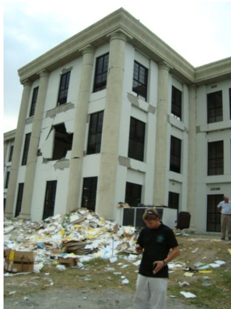
(a) Overall damage including out-of-plane failure of masonry infill wall [06/19/2009, 5:53PM, N15.472899, W88.018565].
