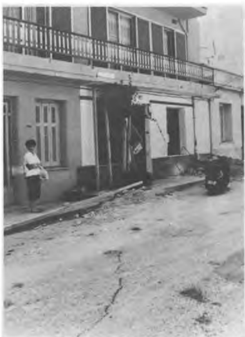
Fig. 7. Structural damage of a two-storey building located on the surface rupture
