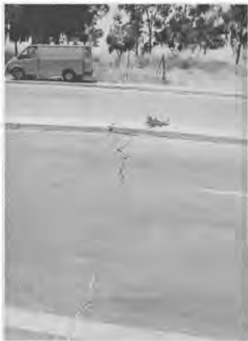
Fig. 2. Surface rupture traced on the pavement of Patras-Olympia motorway
