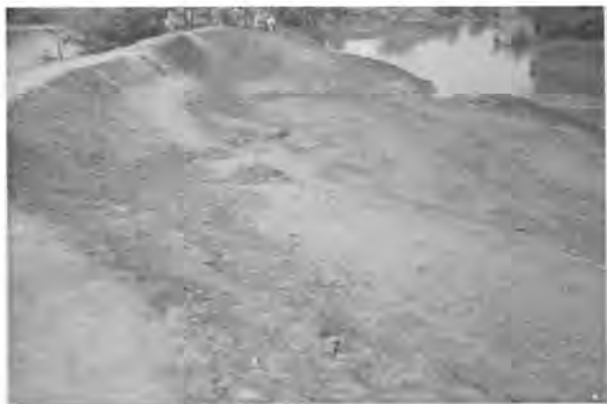
FIG. 7 Subsided Embankment of Kamala River.
