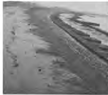
FIG. 6 Longitudinal Cracks on Top of the Bhutahi River Embankment, Zero Nose Near Laukha, Bihar.
