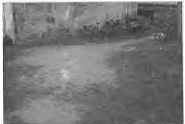
FIG. 4 Sand Boil, Bihar P.W.D. Rest House, Darbhanga.
