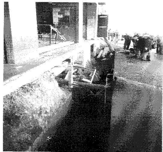
Fig. 6. Large ground displacements around the ferry building on Port Island after the Kobe earthquake, 1995.
