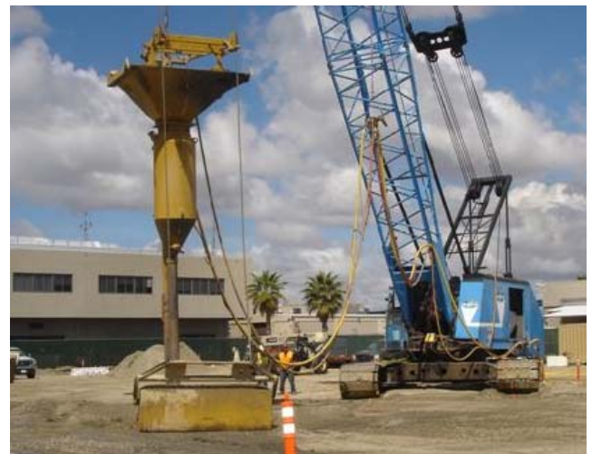
Fig 2. Installation of a Vibro replacement stone column at the storage facility at Naval Amphibious Base in Coronado, CA.
