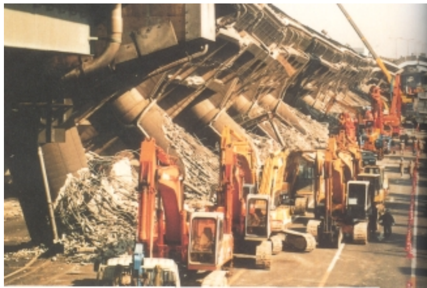
Fig. 1. Partial view of the collapsed bridge
