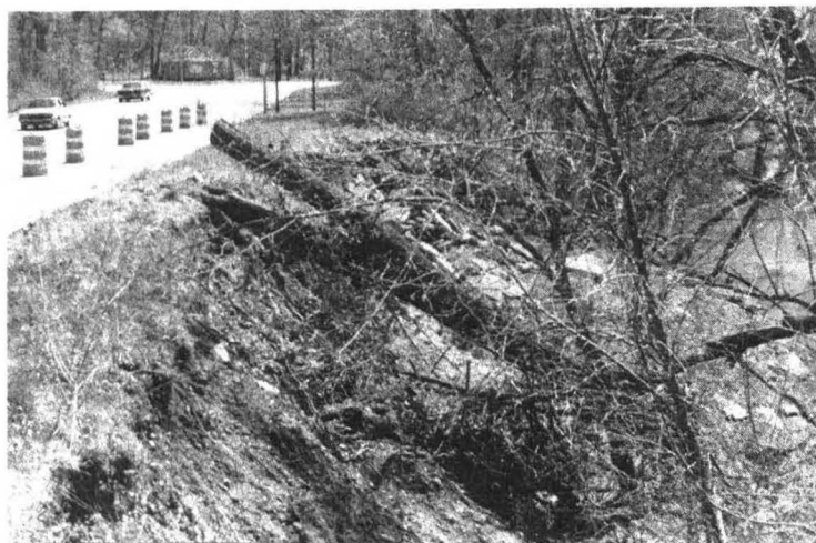
Fig. 4 Existing Channel Bank Slide Location Gregory Blvd. (Blue River Channel)
