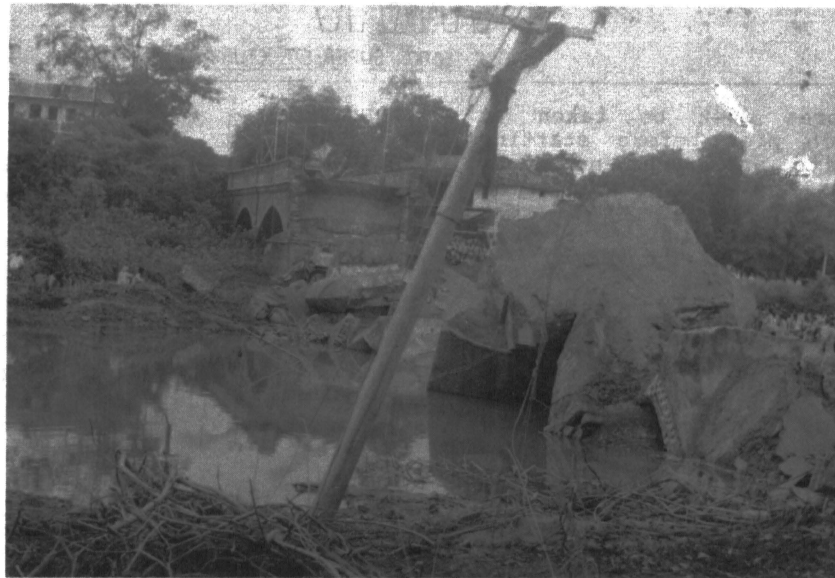
Photo 2. Showing 5 spans collapsed of Palakmati Bridge on Hoshangabad - Piparia Road.
