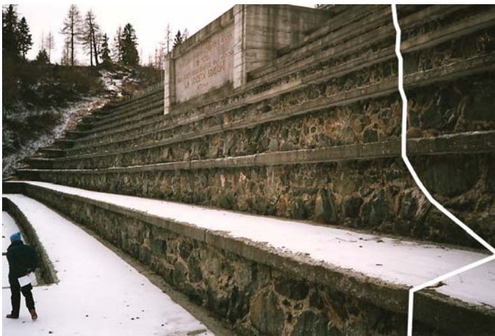
Fig. 4. Down stream abutment of Alpe Cavalli dam with indication of the observed vertical crack.
