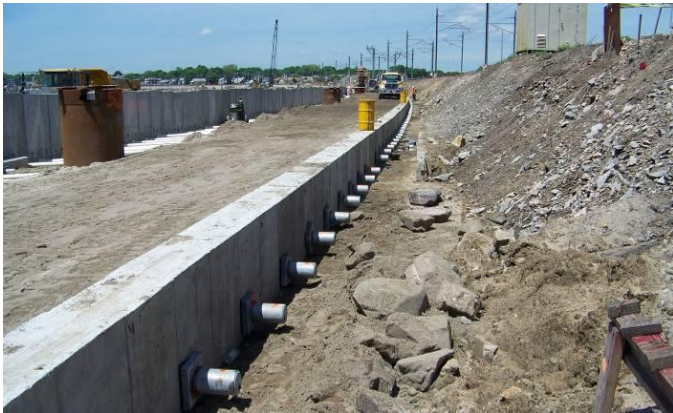
Photo 8. Concrete Deadman with Anchor Rod Protection Cap
