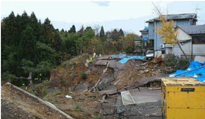
Figure 30: Failure of hillside fill in Takamachi residential area (photo: E. Rathje).
