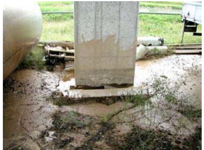
Figure 29: Sand boils at the derailing site of the Johetsu Shinkansen (Oct. 25) (photo: K. Kiyono).
