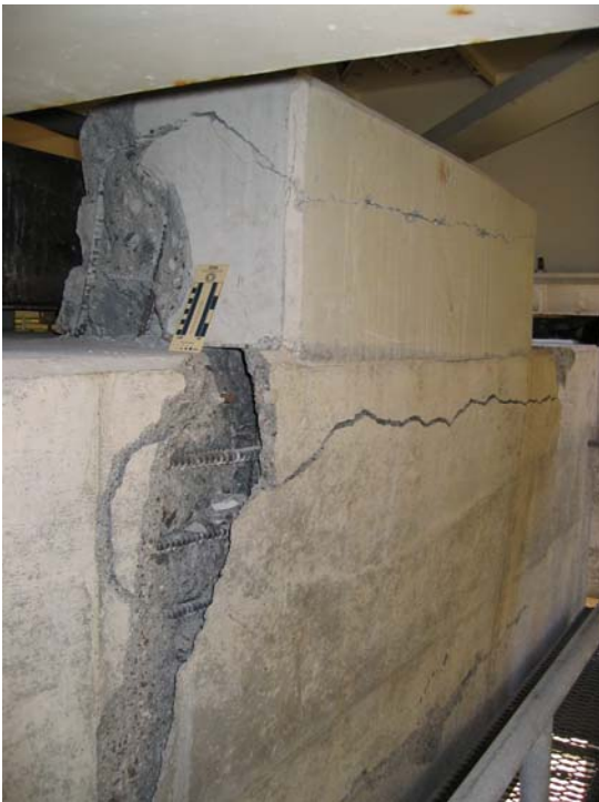
Figure 43. Damaged shear key from the Shizukawa Bridge near Tomakomai City.
