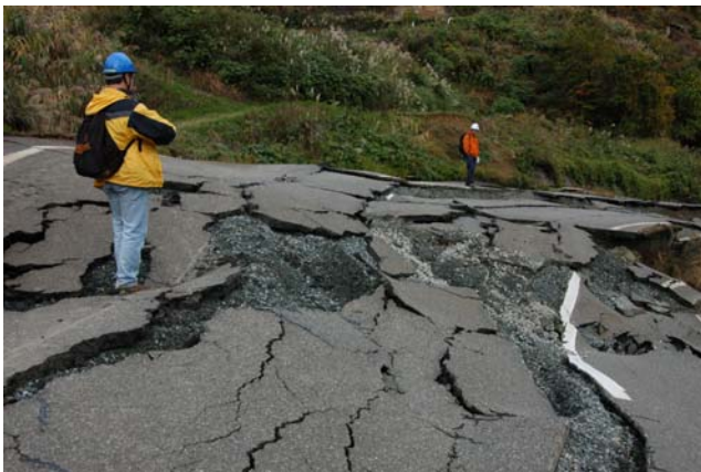
Figure 31: Typical damage to road in Uonoma Hills. (photo: R. Kayen).
