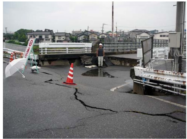
Figure 17: Settlement of approach fill to bridges along the Sabaishi, here, and U Rivers created critical transportation hazards immediately following the earthquake.
