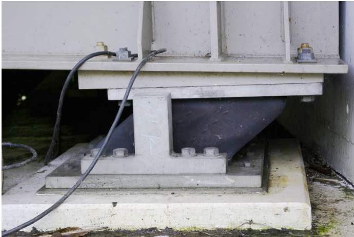
Figure 16: Strained bearing (site SA18, N37.39041° E138.59052°; 7/21/2007)
