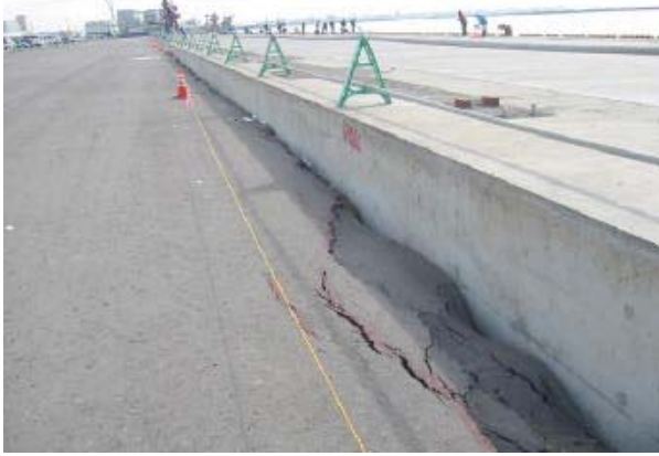
Figure 41. Lateral movement of 10 cm and settlements of 100 cm were observed at Pier 4 of the Port of Kushiro, causing its closure. Piers 1 through 3 suffered minor damage and were quickly reopened.
