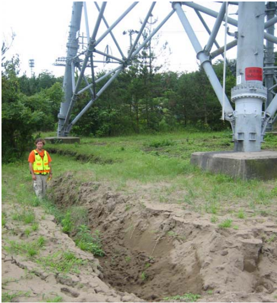
Figure 10: Settlement of ground adjacent to the grade beam between footings of a high voltage transmission line tower (Google Earth map site RK40 - N 37.41633 E138.60792, 7/22/2007).
