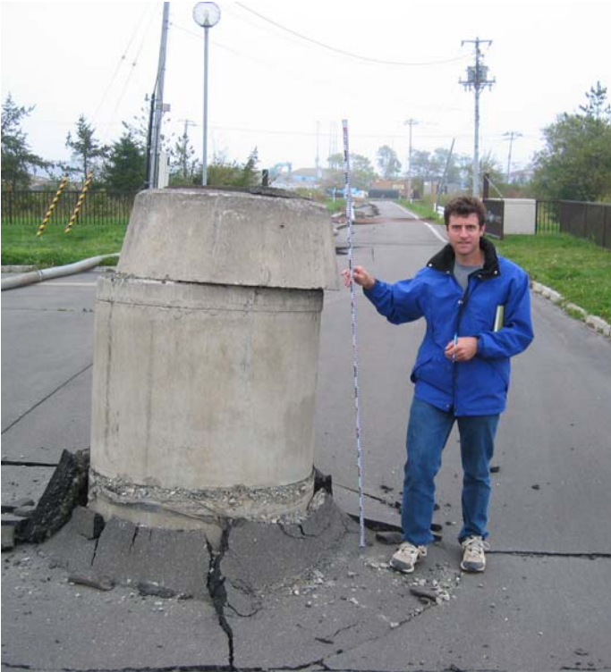
Figure 44. Uplifted manhole near a sewage treatment facility in Otsu town, near the Tokachi river.
