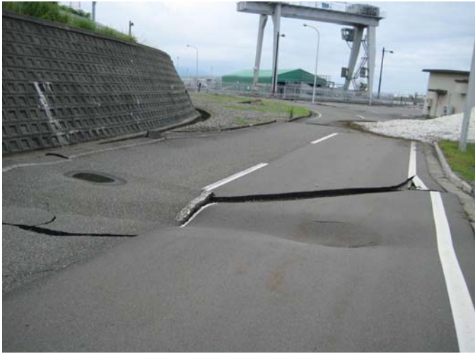
Figure 5: Damaged road at the nuclear power plant (Kayen et al. 2007).
