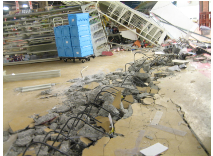
Figure 9: Liquefaction and lateral downslope movement of underlying soil buckled the floor slab of a large warehouse store. (Google Earth map site RK41, N37.41468 E138.60840, 7/22/2007).
