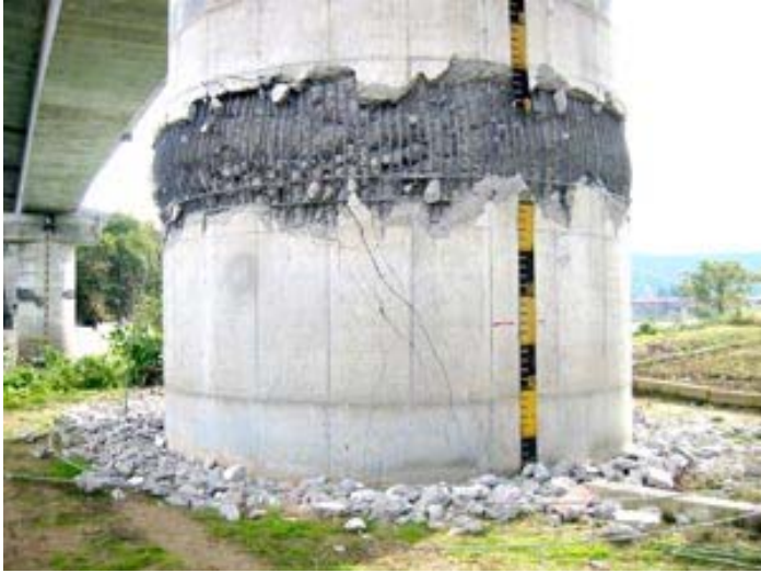
Figure 33: Damaged piers of Joetsu Shinkansen Wanazu Bridge (Nov. 1) (photo: S. Ashford).
