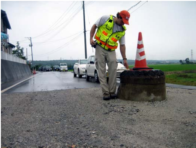
Figure 11: Uplifted manholes from storm-water drains impeded traffic and compromised rainfall drainage throughout Kashiwazaki City and the surrounding villages.
