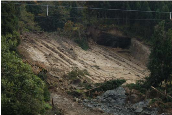
Figure 27: Block slide formed by bedding plane (sliding surface) and two sets of vertical joint release surfaces (photo: R. Kayen).
