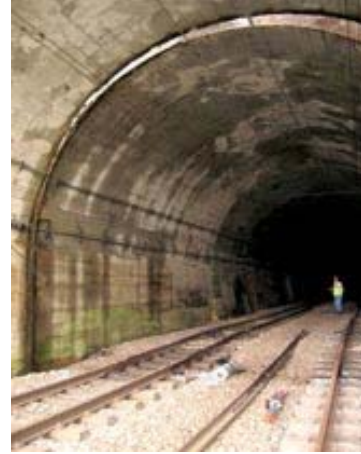
Figure 35: Photograph (below) and LiDAR image (above) of damage to the Juetsu Railroad portal at Kita-Horinouchi from the portal entrance. Lateral displacement of the portal in the photo is visible and measurable in the LiDAR scan. (: R. Kayen)
