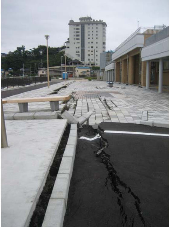
Figure 20: Kashiwazaki Harbor – Liquefaction induced lateral spreading and settlement of soil beneath a harbor-front caisson resulted in rotation toward the harbor and lateral displacement of the soil behind it (Site RK25, N37.36713 E138.53210, 7/20/2007).
