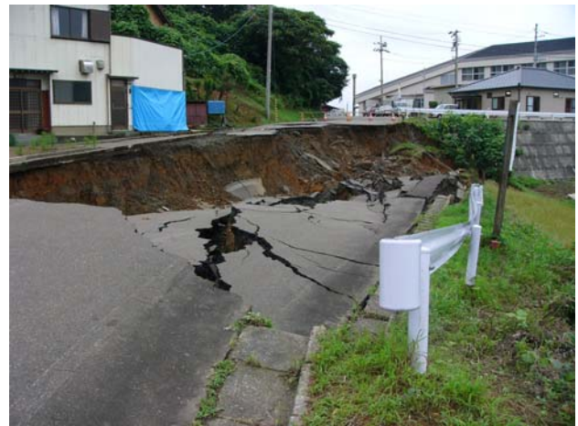
Figure 14: Road embankment failure off Route 8 on the way to Kasashima (Site YT18; N 37.33325 ° E 138.46500°; Photo taken 7/21/07)
