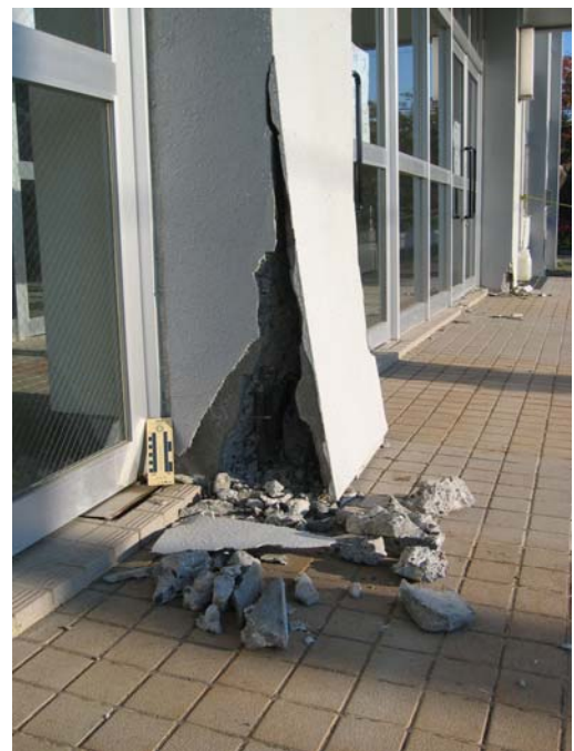
Figure 42. Damage to Urakawa Elementary School.
