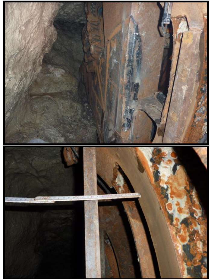
Fig. 6. Cutter Head damage, Esfahan Subway Project, Eastern Tunnel
