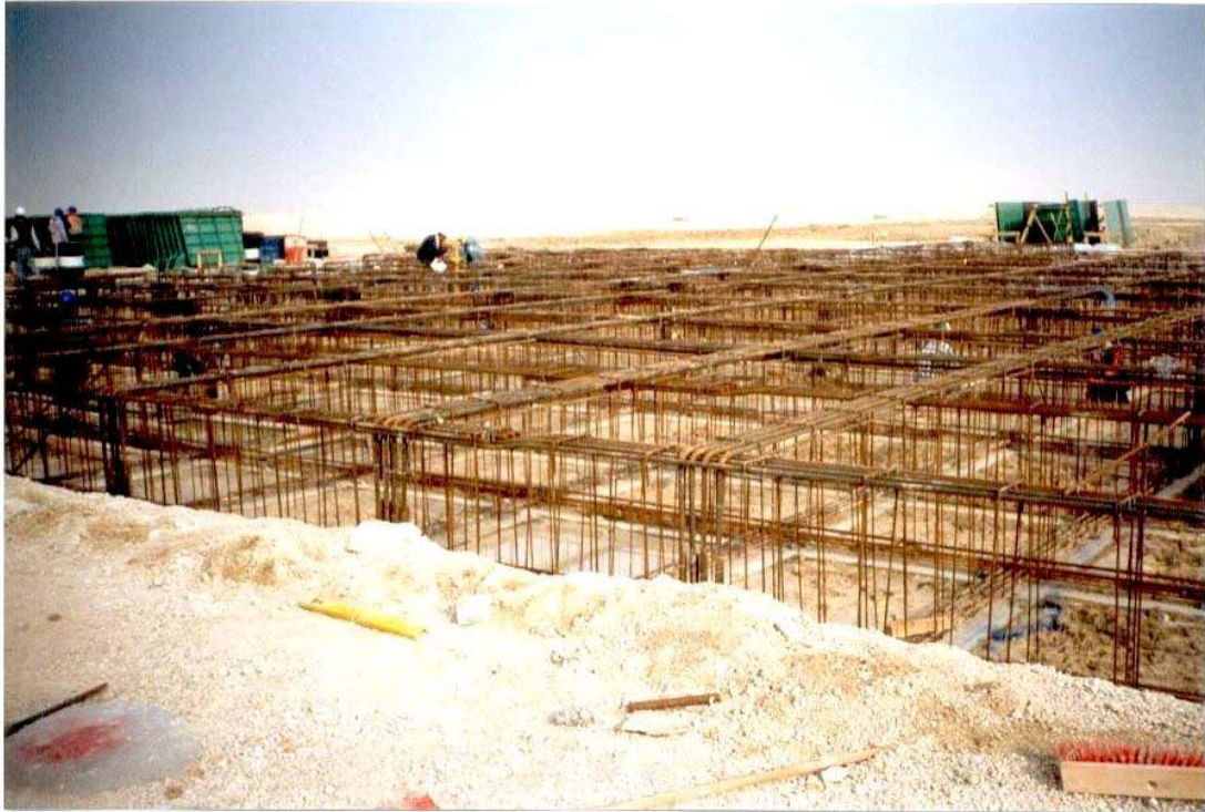
Plate: 1 Excavation & Rebar placing for Stiffened Slab Waffle Foundation at the Site
