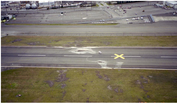
Fig. 6. Liquefaction ejecta in runway and sink holes in adjacent field, King County International Airport
