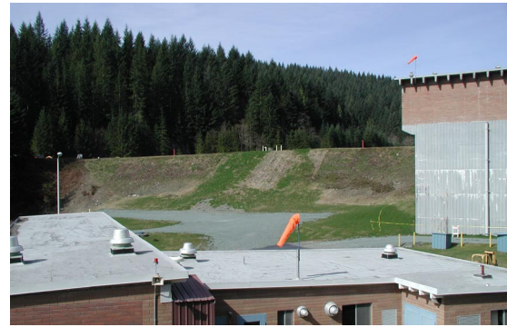
Fig. 7. Lake Chaplain South Dam, toe area to the west (left) of the inlet tower improved with vibro-replacement stone columns
