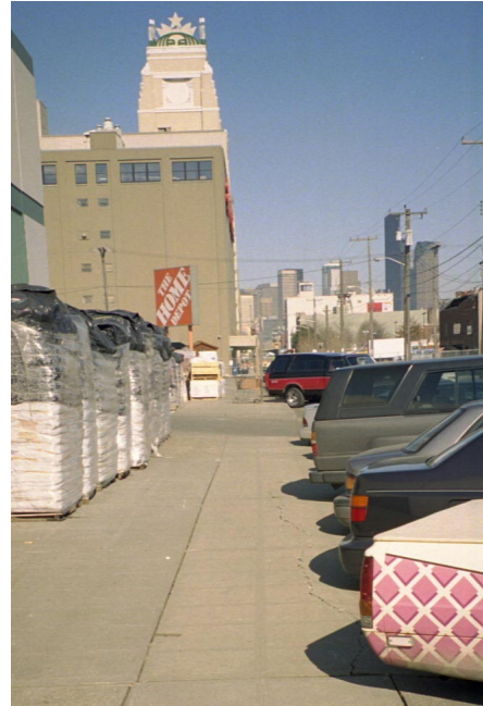
Fig. 3. Crack in sidewalk along east side of Garden Center, looking north, outside improved zone
