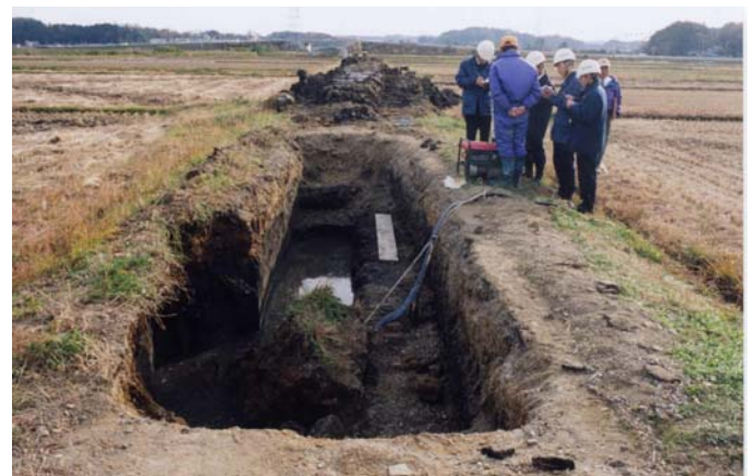
Fig. 2. Labor accident caused by trench collapse.
