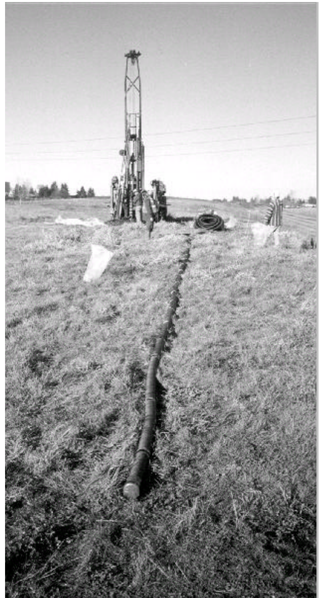
Fig. 3 Corrugated ABS extensometer pipe at instrument station B-6, with attached settlement rings.
