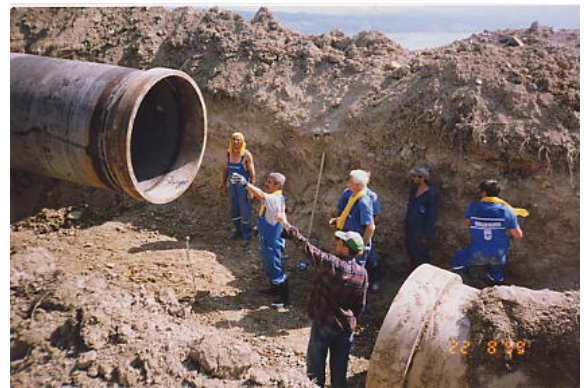
Fig. 3. Repair and replacement studies on damaged AC pipeline after earthquake.
