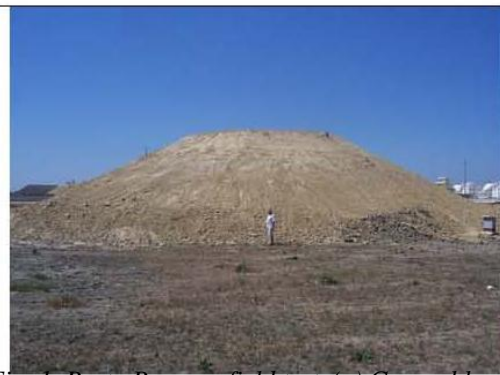
Fig. 1. Porto Romano field test. (a) General location of the site, (b) Photographs illustrating the failure of the embankment at day 18 from the start of construction, (c) Photograph of the embankment at top height
