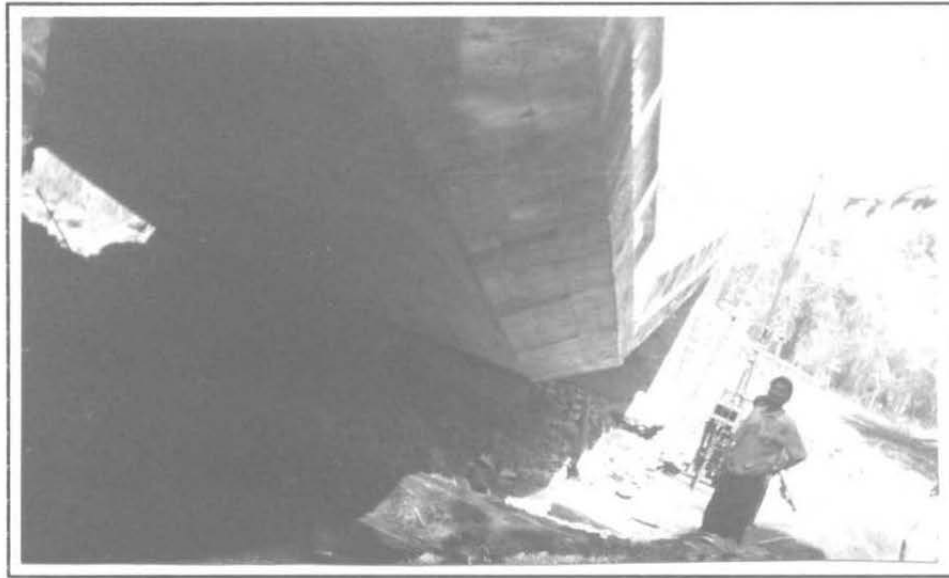
Photograph 1 View showing the collapse of pier
