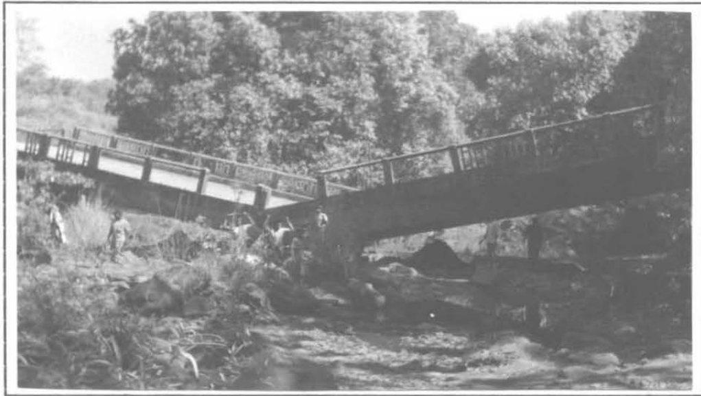
Photograph 3 View showing deck slab resting on bed level with no damage signs
