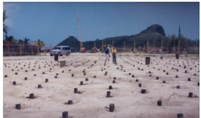
Fig. 8. Photograph of drain installation at Hyatt Regency Hotel and Casino prior to installation of piles.
