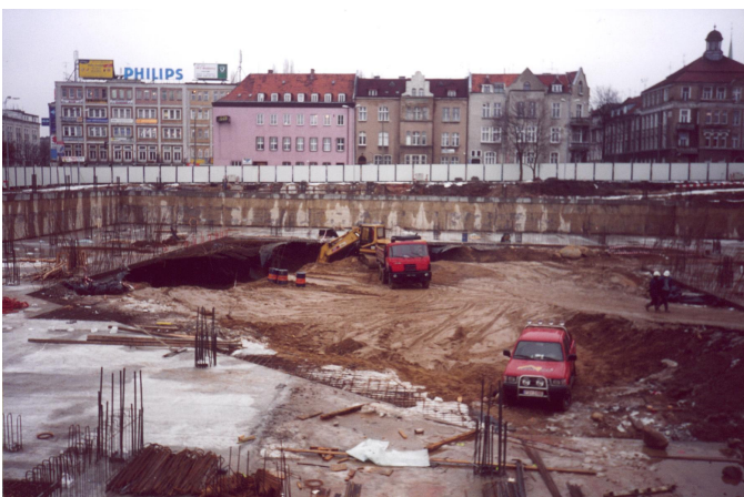
Fig. 5. General overview of excavation at “-1” level stage. The “-1” parts of permanent floor slabs (the rest of floor has been carried out in further phase of works).
