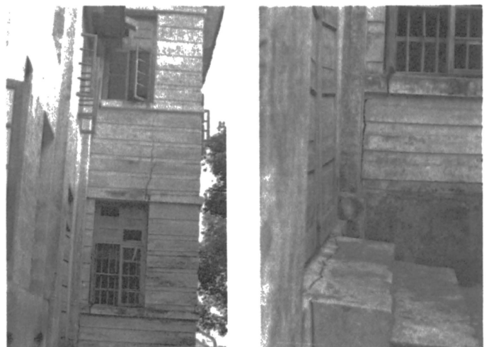
Fig 9. Crack Damage To A Two-storey House Caused By Ground Crack.
