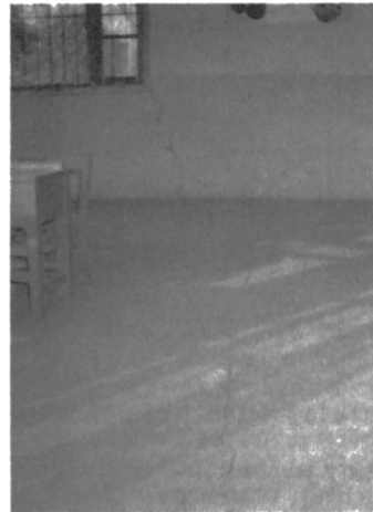
Fig 8. Crack Damage To A Single-storey House Caused By Ground Crack
