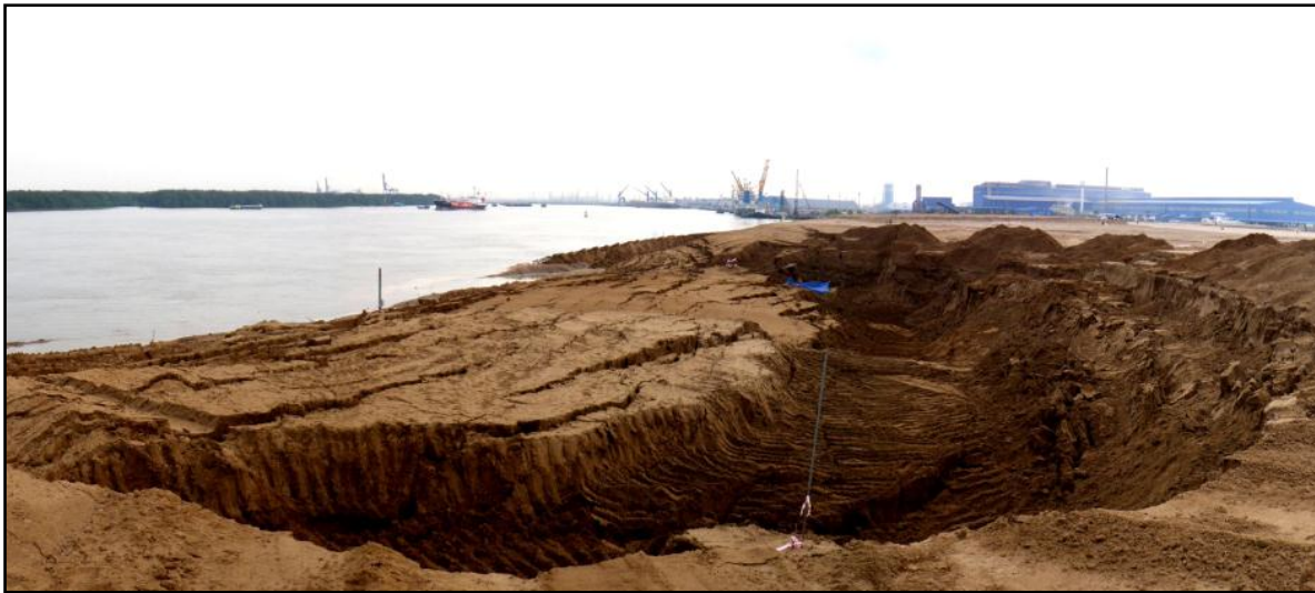
Fig. 2 Slope failure on July 12, 2010, viewed upstream
