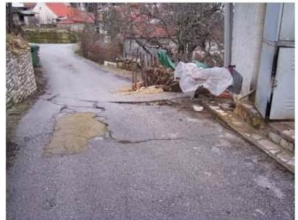
Fig. 6. Kerasia slide. Photos at 28/12/2010. (a) . Typical damage at house. (b). Damage at wall illustrating differential movement. (c). Differential movement at road
