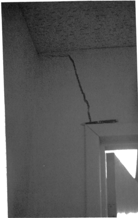
FIG. 1. Typical Damage to the Building Wall
