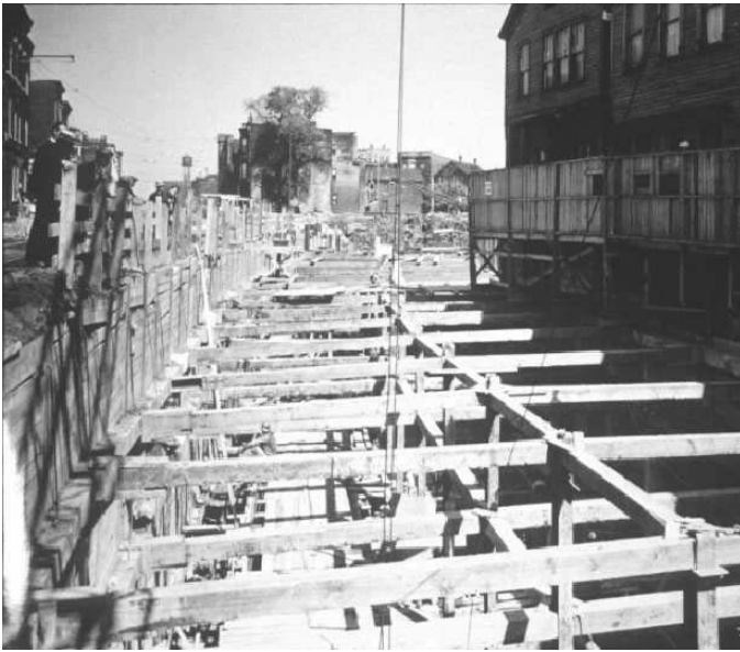
Fig. 2. Braced open cut on Contract S-1A of the Chicago Subway, as seen in July 1940. This view shows the transition between the elevated and below ground sections of the State Street line, towards its north end, near the intersection with Clybourn Avenue.
