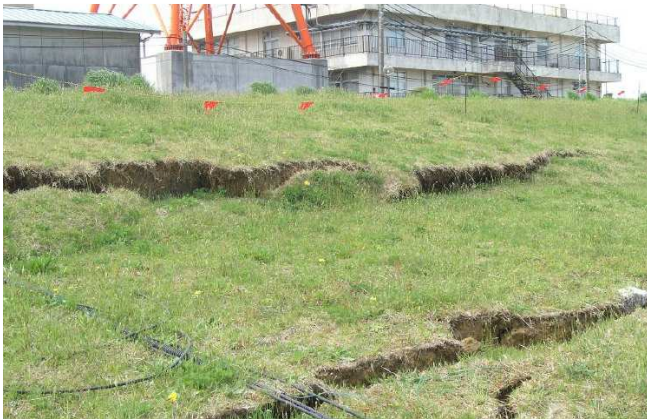
Fig. 1. Liquefaction-induced distortion of Tone river levee in Sawara (Towhata et. al 2011)
