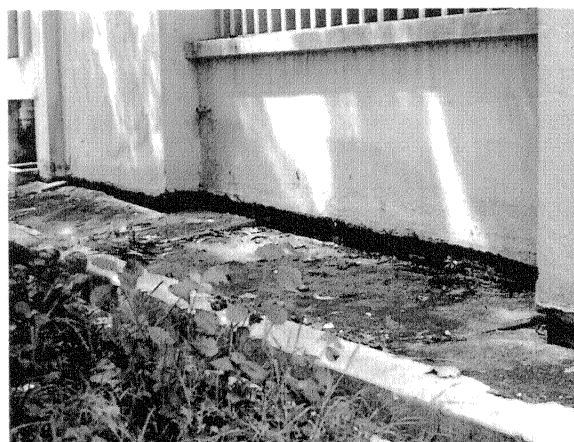
Fig.4 Settlement of skirting
