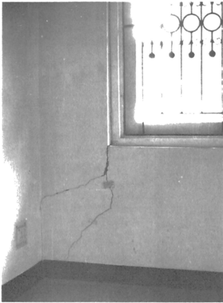
Fig. 7 A typical crack
