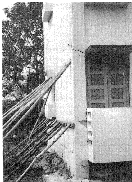
Fig. 3 Cracks in a three storeyed building in Madras
