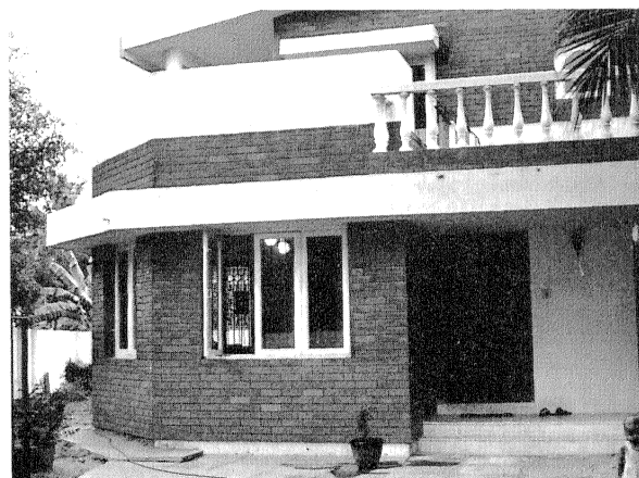
Fig. 6 Single storeyed portion of building which developed cracks
