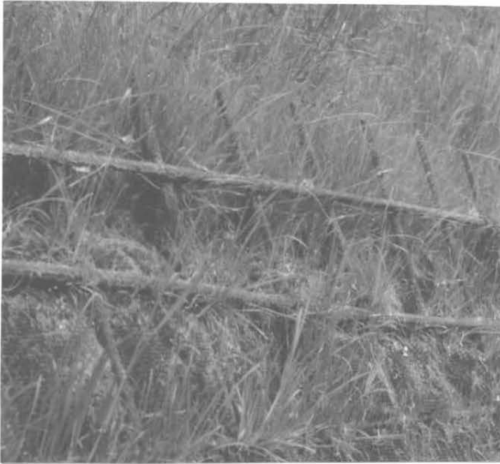
Photo 4: local view of the facing 8 months after
