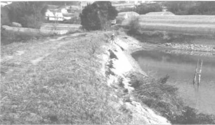
Photo. 3 Damaged earth dams of Grade 3 (Ichinomiya-cho in Awaji Island)
