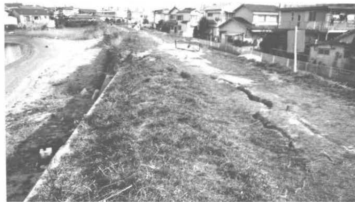
Photo. 4 Damaged earth dams of Grade 2 (Akashi City in Honshu Island)
