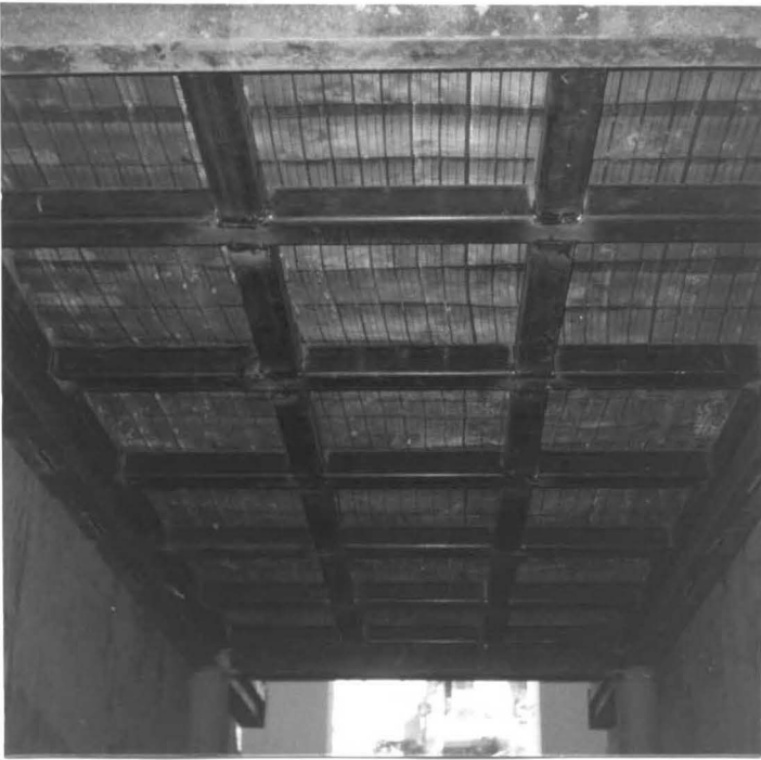
Fig. 3 Grid system under wooden floor
