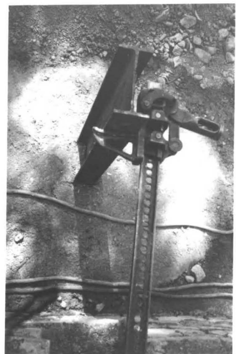
Fig. 5 Jacking force for the stiffener
