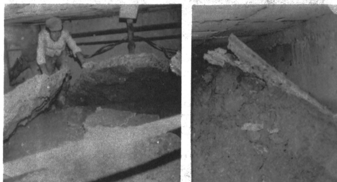
Fig.2 The rejected soil in the basement rooms toward the large settlements area
