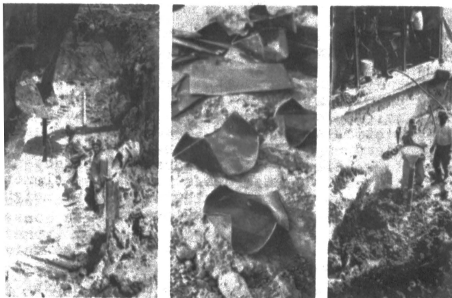
Fig.7 Thrust of vertical pipes used to introduce quick lime in the foundation ground (a). Metal sheet bent at corners (b)
