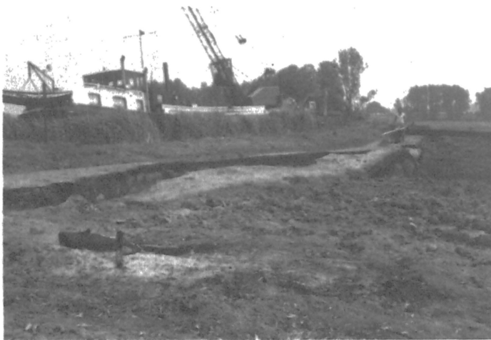
Fig. 5 Sliding of the innerslope of the dike
